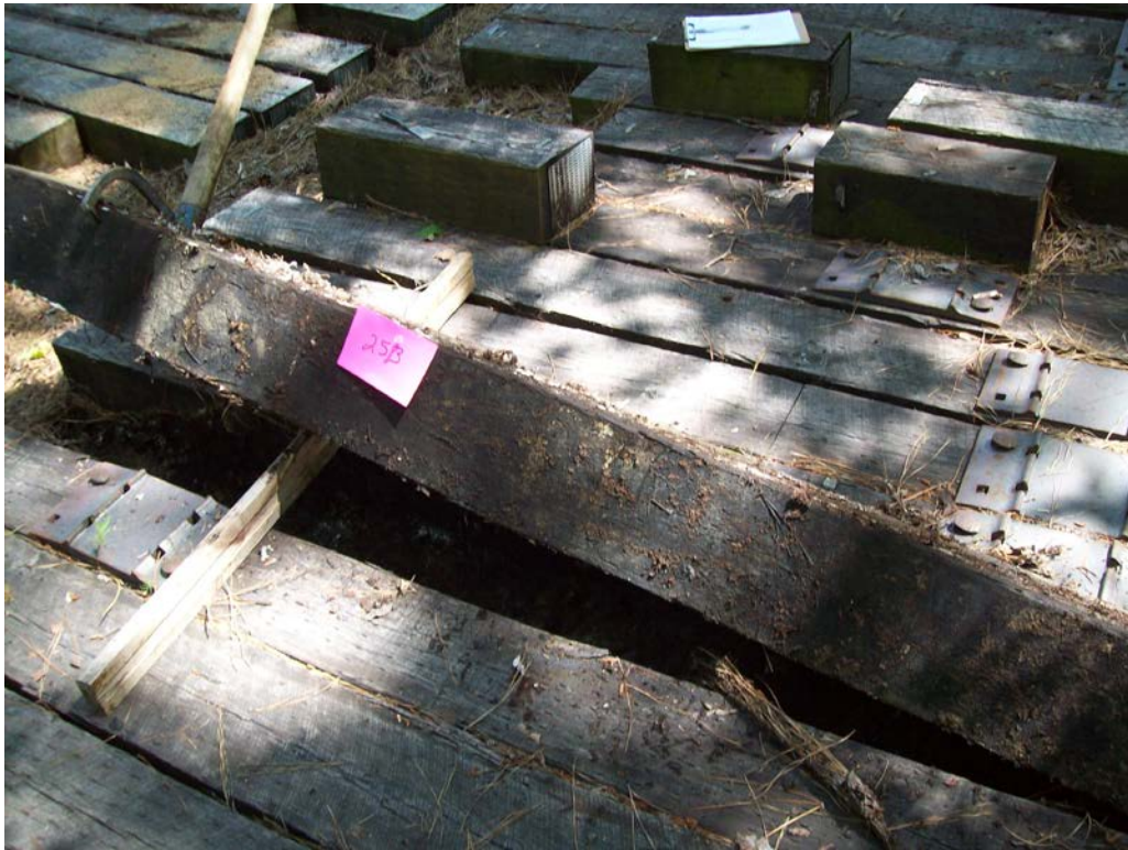
Figure 501 - Tie #253 (Koppers/white oak/creosote petroleum solution).
