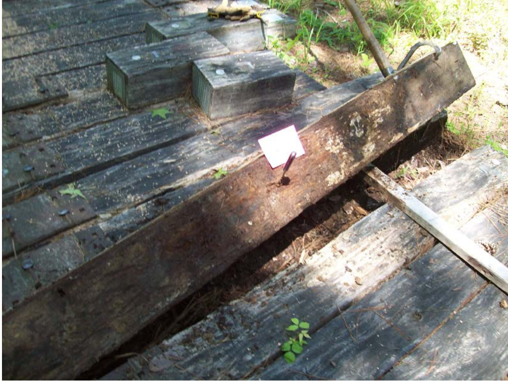
Figure 41 - Tie #208 (Nisus/white oak/borate) with decay on bottom.
