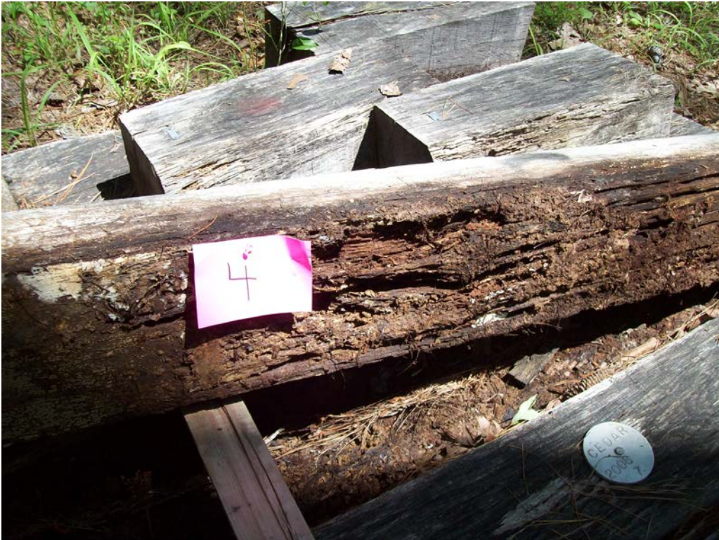
Figure 1 - Tie #4 (Cedarcide/white oak) with decay.
