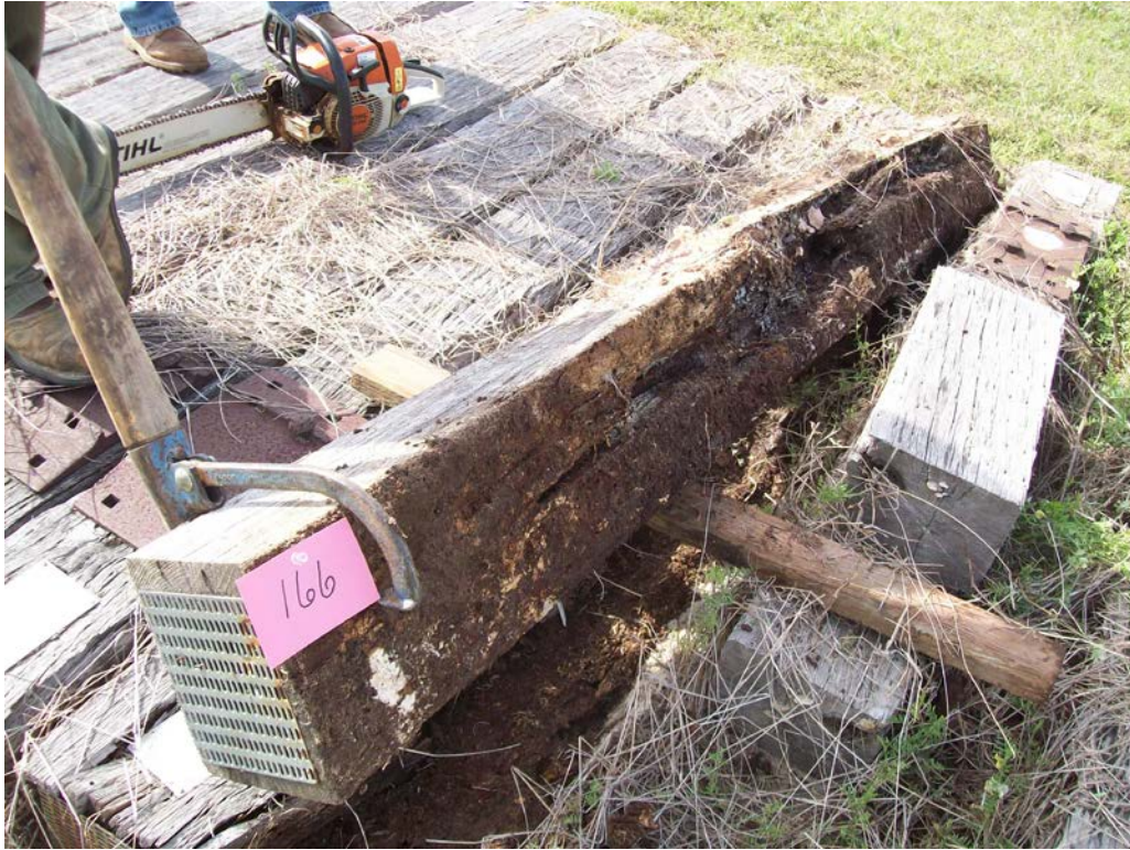
Figure 29 - Tie #166 (untreated/White oak) with extensive decay.
