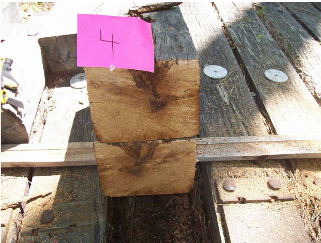
Figure 2 - Tie #4 (Cedarcide/white oak) with decay.
