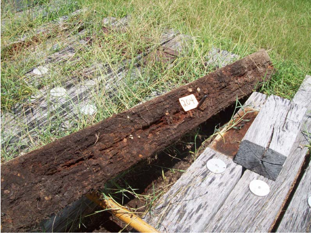
Figure 39 - Tie #204 (Cedarcide/red oak) decay on bottom and side.
