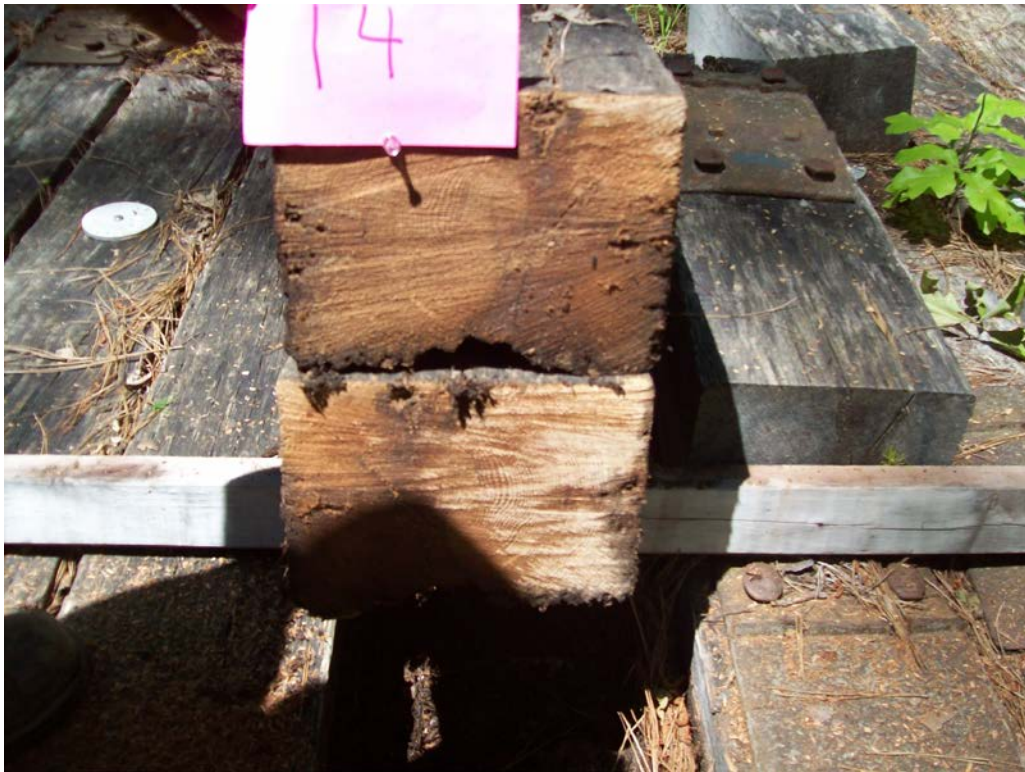
Figure 4 – Tie #14 (Cedarcide/red oak) with decay.
