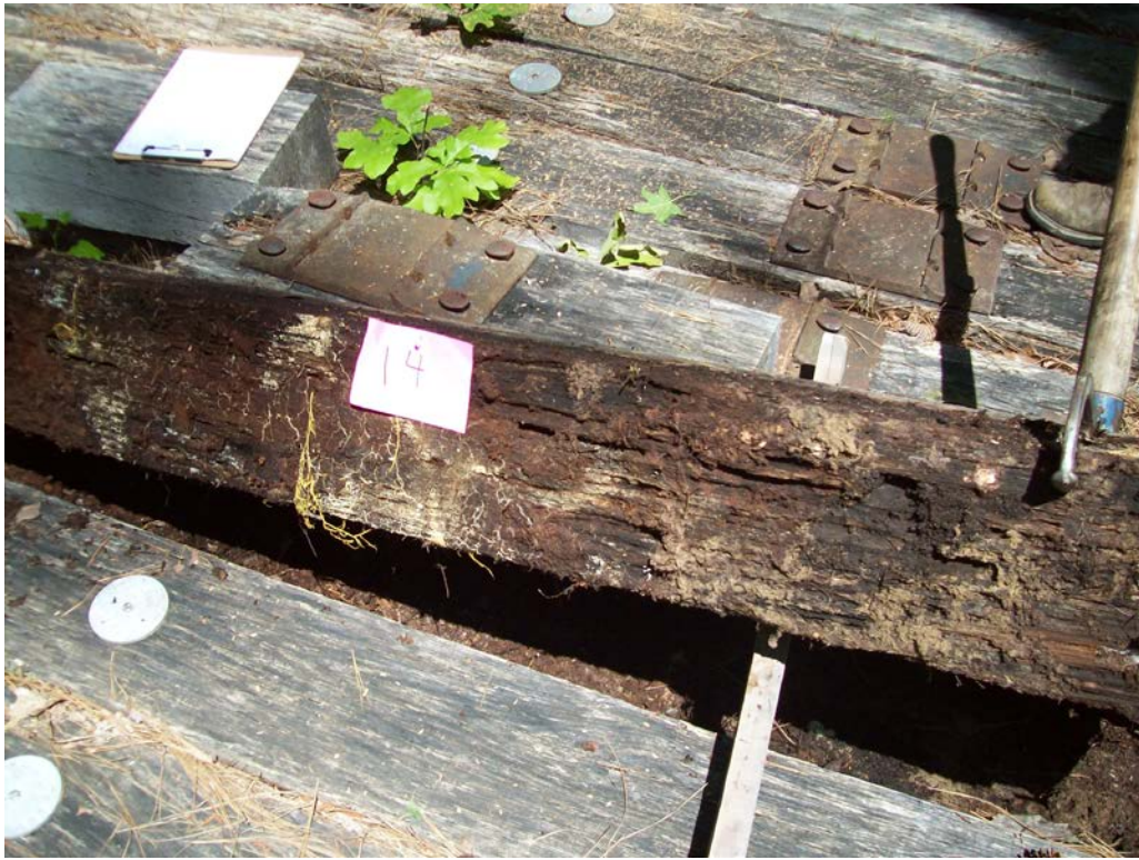
Figure 3 – Tie #14 (Cedarcide/red oak) with decay.
