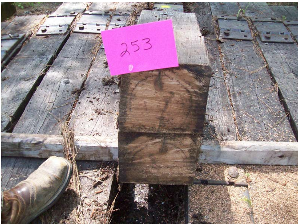
Figure 512 - Tie #253 (Koppers/white oak/creosote petroleum solution).
