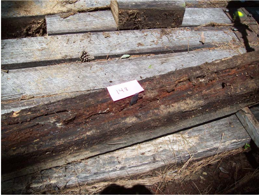
Figure 29 - Tie #148 (untreated/red oak) with extensive decay.
