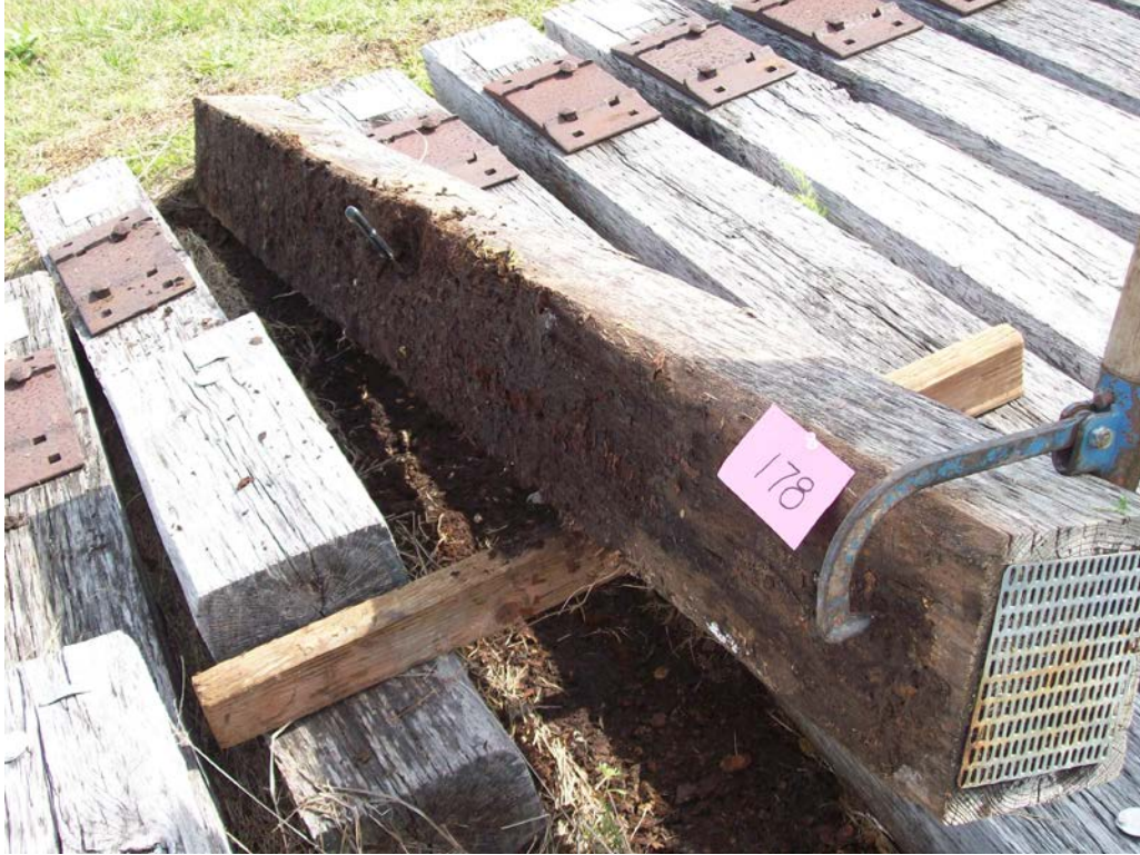
Figure 33 - Tie #178 (Lonza/red oak) with decay evident.
