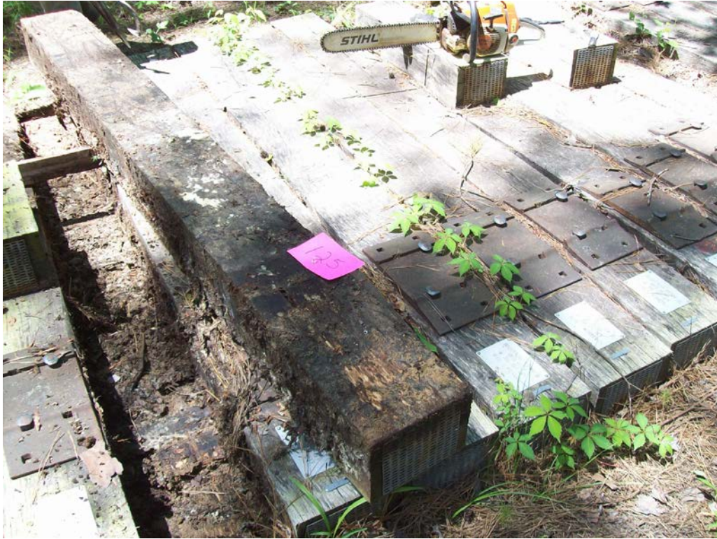
Figure 23 - Tie #125 (Lonza/red oak) with light decay on bottom.
