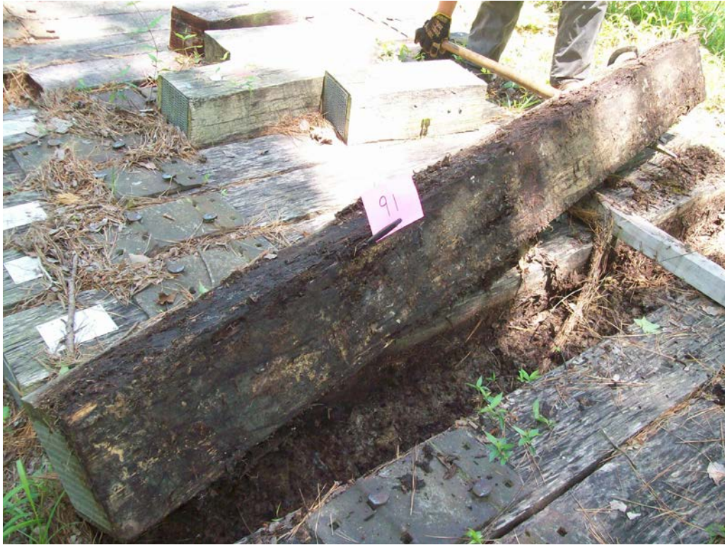
Figure 17 - Tie #91 (Lonza/white oak) decay on bottom.
