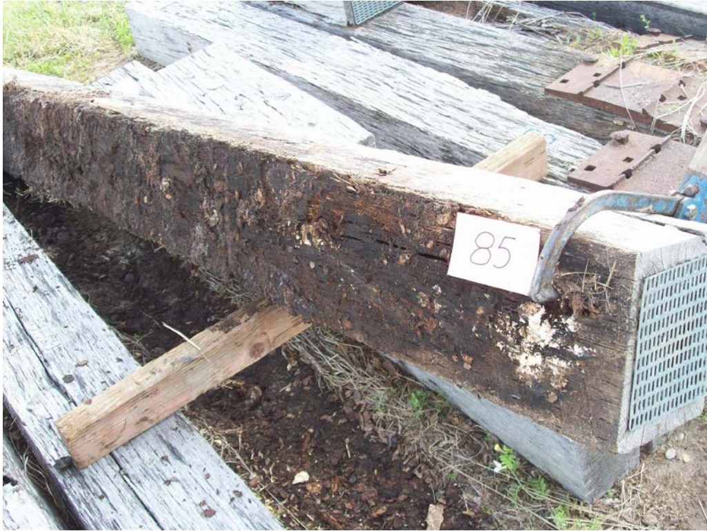
Figure 17 - Tie #85 (Lonza/red oak) decay on bottom.
