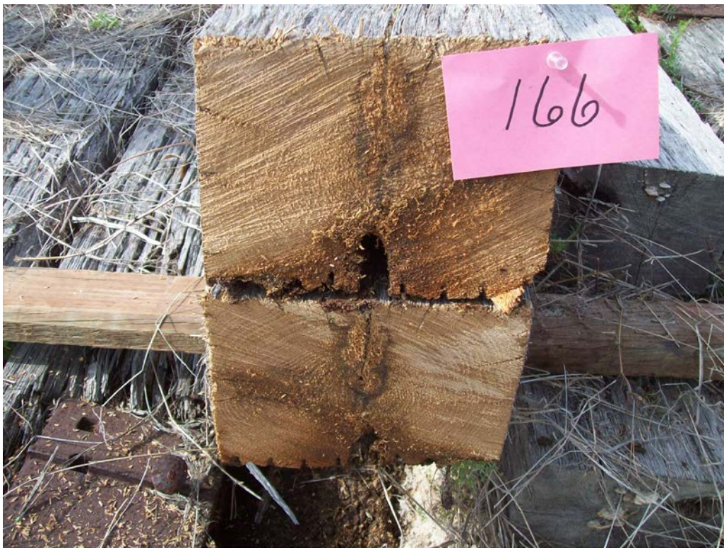
Figure 30 - Tie #166 (untreated/white oak) with decay.
