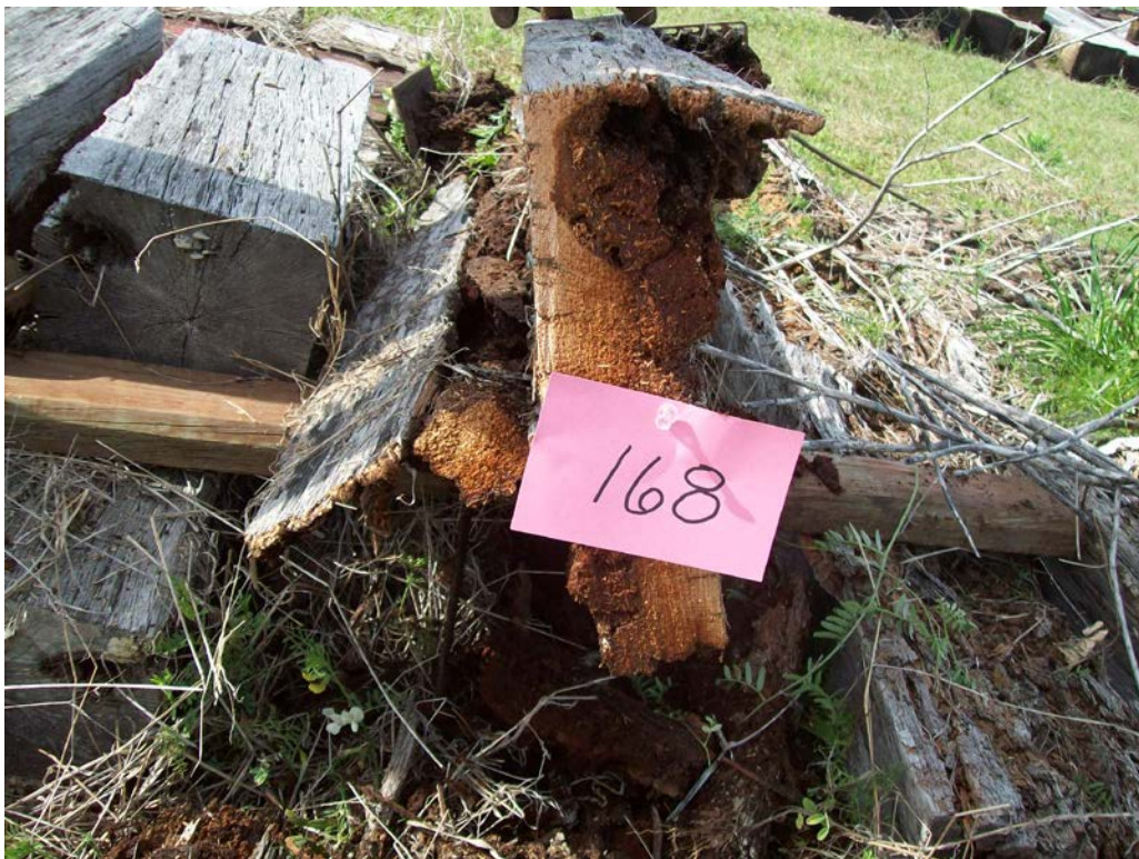
Figure 32 - Tie #168 (untreated/red oak) complete failure.
