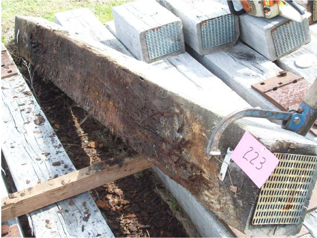
Figure 43 - Tie #223 (Merichem/red oak/CuNap) with light decay.
