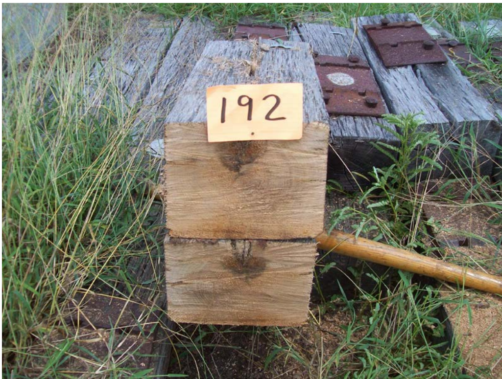
Figure 38 - Tie #192 (Cedarcide/white oak) internal decay.
