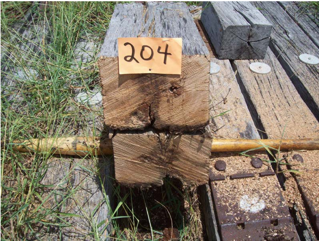
Figure 40 - Tie #204 (Cedarcide/red oak) internal decay also.
