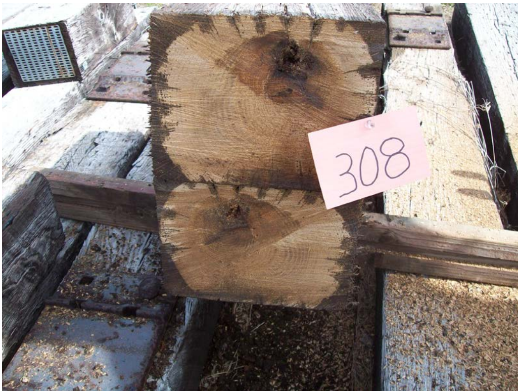
Figure 534 - Tie #308 (Koppers/white oak/creosote petroleum solution) with heart decay.
