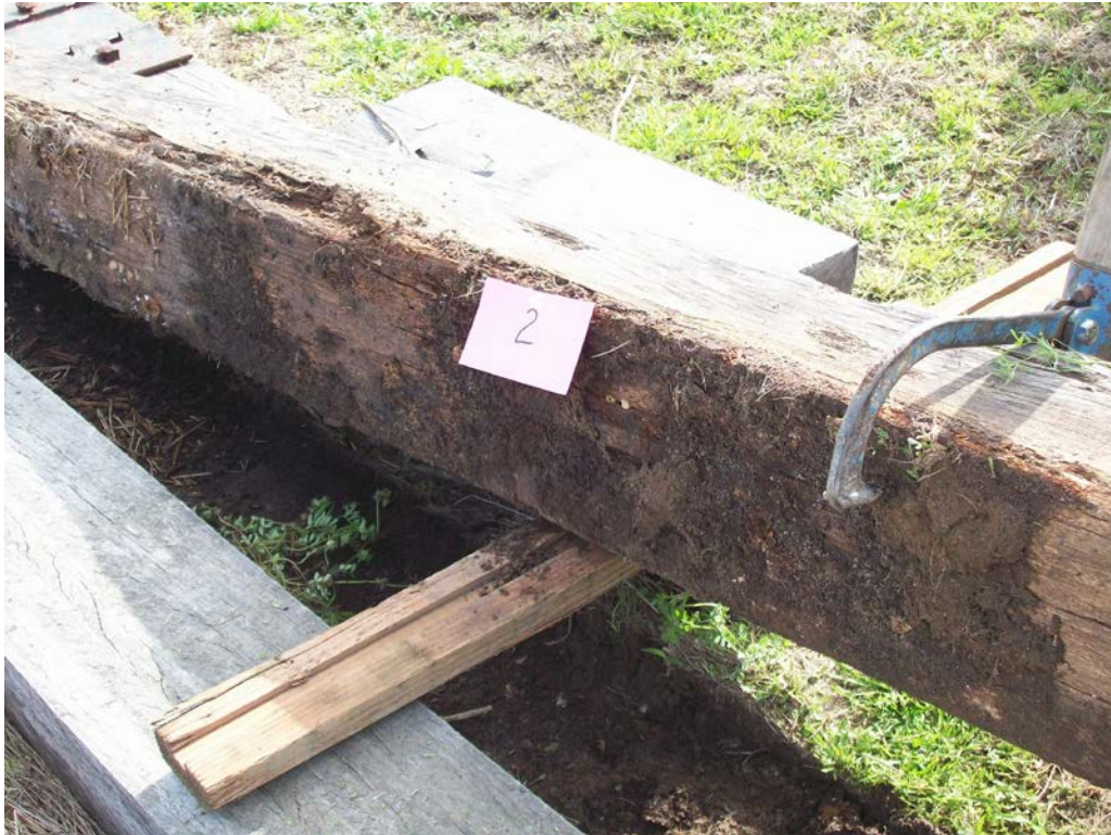
Figure 1 - Tie #2 (Turada) with decay.
