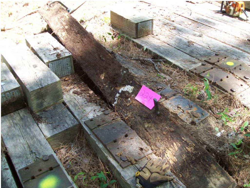
Figure 45 - Tie #224 (untreated/white oak) with decay.
