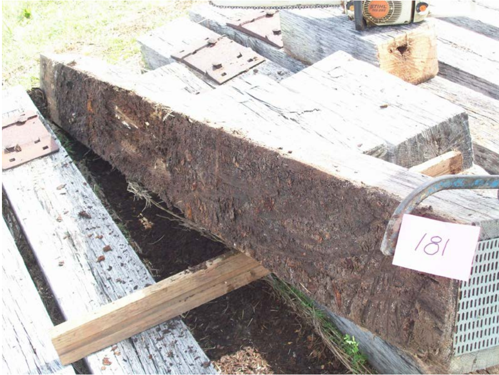
Figure 35 Tie #181 (Lonza/white oak) with decay on bottom.
